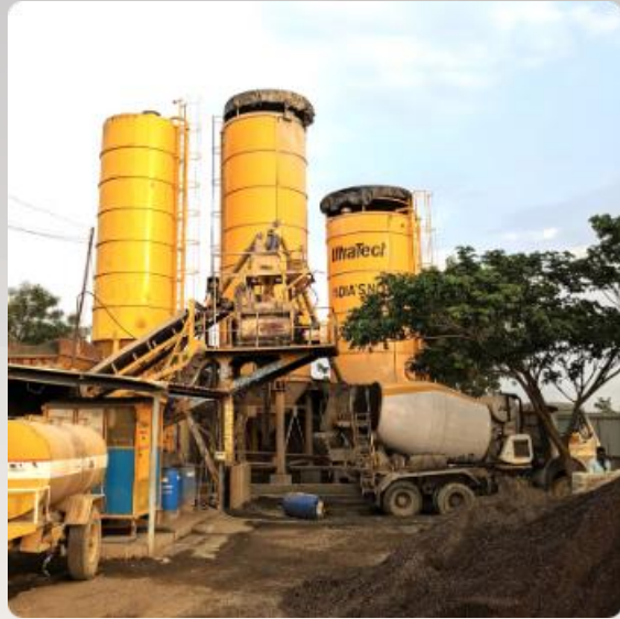
Concrete Batching Plant Plant
